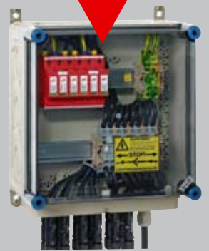
PV generator junction boxes
